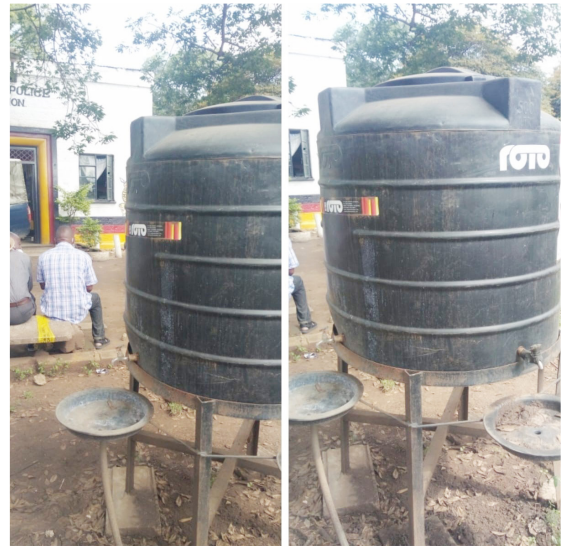
▶ 500 litres ROTO handwash station donated to Makongeni Police station
